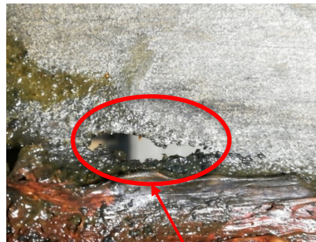
Failure after 20 cycles
